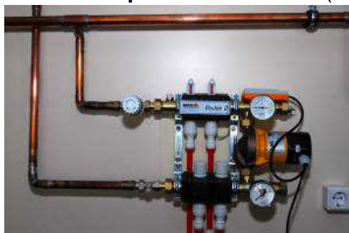
Illustration 10a: Wrong – insulation lacking on the entire piping system
